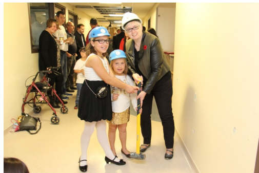
Photo Above: Gabby and Daniella Pizzuti, along with Margaret Anderson, Executive Director, RMHSWO begin the demolition process during a ceremony to officially start construction on 3West.
