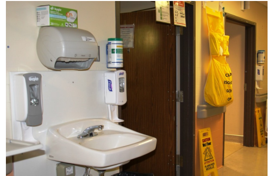
PHOTO ABOVE: Clearly labelled and defined PPE (Personal Protective Equipment) including gloves and gowns on one side of the door and hand hygiene and wipes on the opposite side, conveniently located between patient rooms; a standard to be expanded to other areas and floors.
